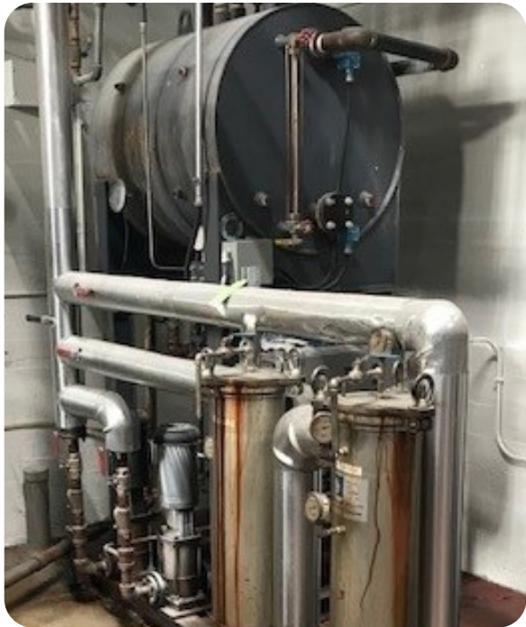
The condensate return equipment pictured here in our Guelph facility captures and recycles steam condensate, reducing energy consumption and water usage. By improving thermal efficiency, the project not only lowers operating costs but also supports our goal of achieving net-zero emissions by 2050 by reducing annual emissions by 180t CO 2 e.
